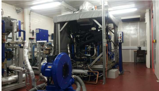
Engine test cell
